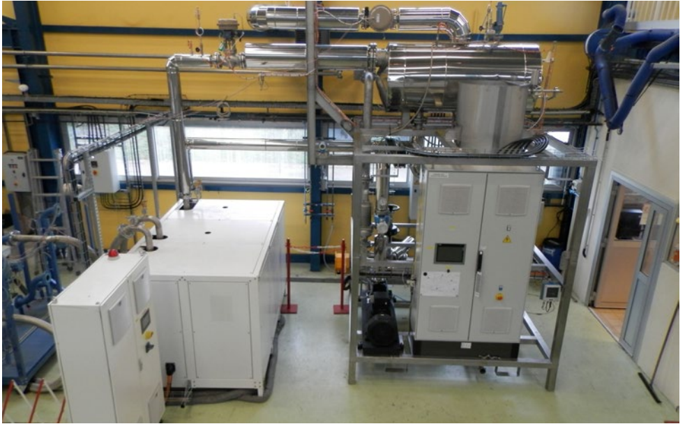
Figure 2. Demonstrator of the steam-generating heat pump employing a flash tank realized within the BAMBOO project.
